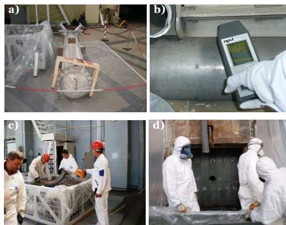
Figure 4. Categorization of RAW: a) intermediate storage of dismantled equipment, b) measurement of gamma dose rate, c) RAW sorting, d) dismantling of the thermal column
