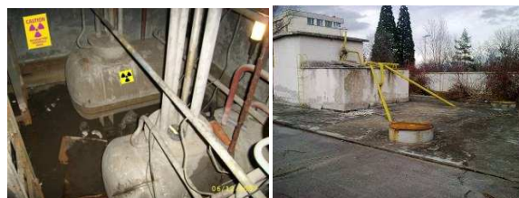
Figure 6. Liquid RAW storages: Left-LRAWSlv, Right-LRAWSHv
